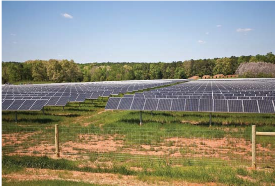
The 1 MW solar array at SAS's headquarters in Cary went live in December 2008, contributing to the six-fold increase in North Carolina's installed solar power in 2008. Many projects like this one are scheduled to go online in the next two years, including another 1.2 MW installation at SAS. 42
